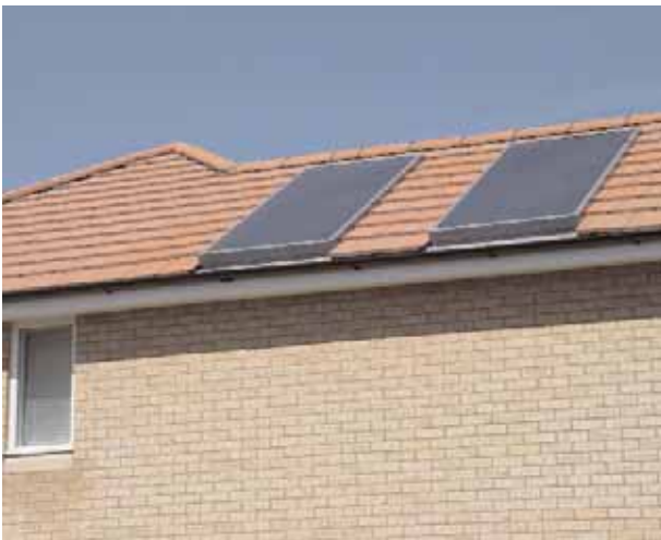
Solar water heating panel in Milton Keynes
