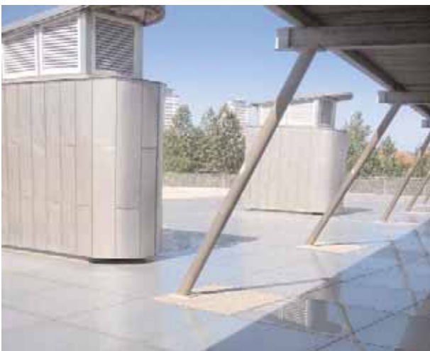
Ventilation stacks at the National Glass Centre are an integral part of the design of the building
