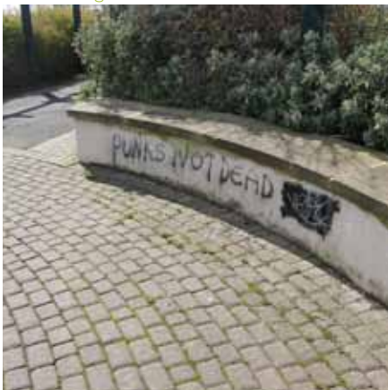
Evidence of graffiti
