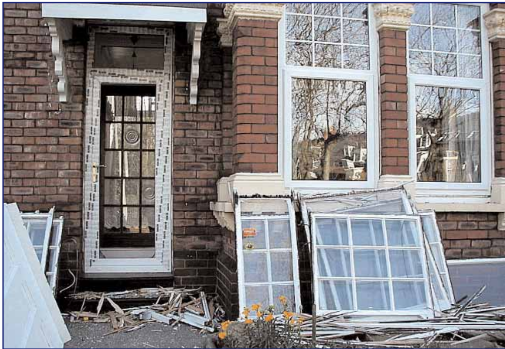
The installation of UPVC units, as illustrated above, fail to match the slender proportions and detailing of the traditional sash windows, detracting from the character of the property concerned and the terrace as a whole.
