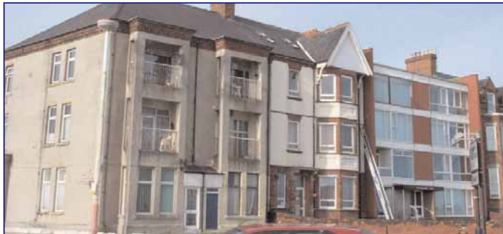
The above property, prominently located at the southern end of Roker Terrace, has been substantially altered from its original form and is in a state of disrepair. This is an unfortunate sight at the main gateway into the Conservation Area from the south and portrays a negative image of the area.
