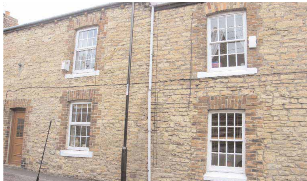
This photograph of Garden Street illustrates the difference in quality between original timber sliding-sash windows, shown to the right, and uPVC replacements to the left. The stick-on glazing bars, shiny material and thicker sections and lack of depth of the frames of the uPVC units provide a poor imitation of the original windows and detract from the historic character of the terrace.
