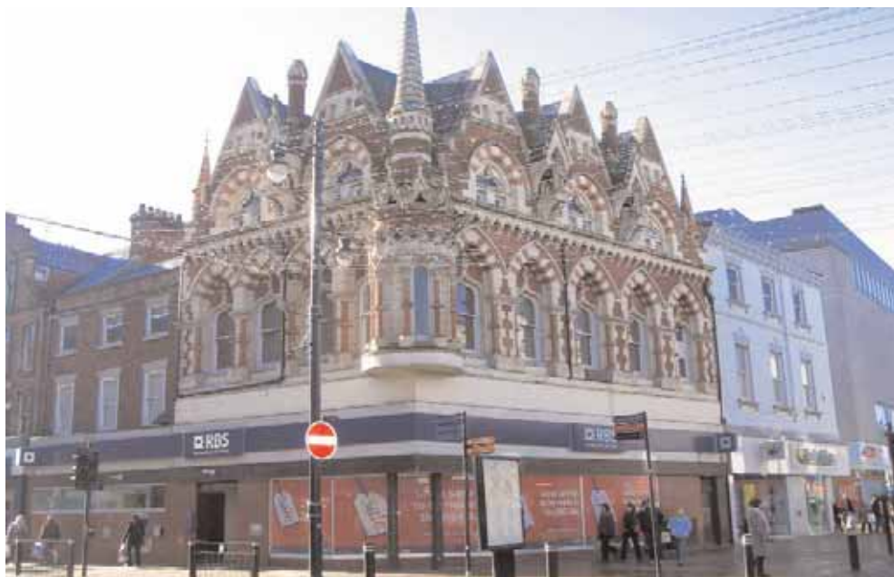
The features and architectural detail of the upper floors of the Royal Bank of Scotland (former Elephant Tea Rooms) are unique and exceptional, but are in need of some essential maintenance to remove plant growth, for example, which can be very damaging to the building's fabric and features. Although upper floors do not present active frontages to the shopping parade and are not publicly accessible, it is nonetheless essential that the high quality upper floors of such buildings are not ignored and are suitably conserved and maintained into the future.
