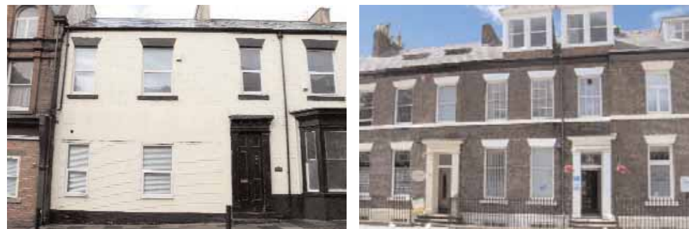
Above: uPVC windows in an historic property (left) fail to accurately reflect the elegant proportions of traditional timber sliding sash windows (right).
