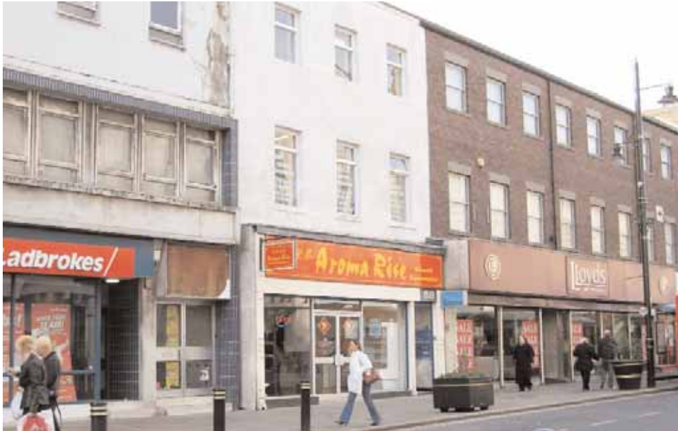
Poor quality modern shop frontages on Fawcett Street. The property on the left can also be seen to be suffering from a lack of maintenance above ground floor level.
