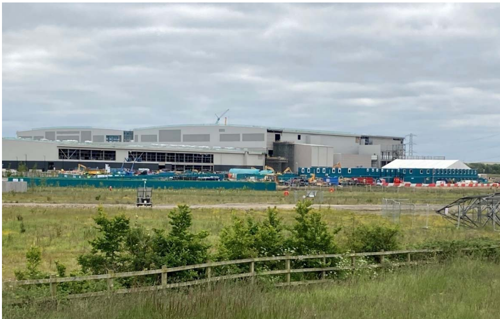
Figure 2.3 Photograph of the battery plant being constructed – taken from the site car park
