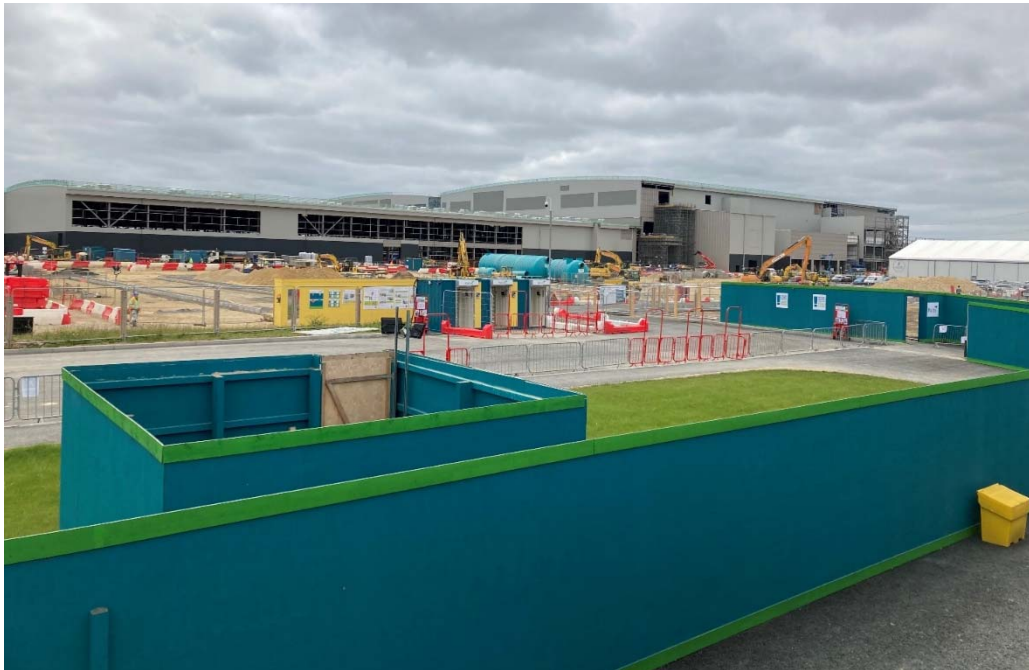
Figure 2.2 Photograph of the battery plant being constructed taken from the site compound
