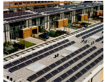
The use of photovoltaic cells
