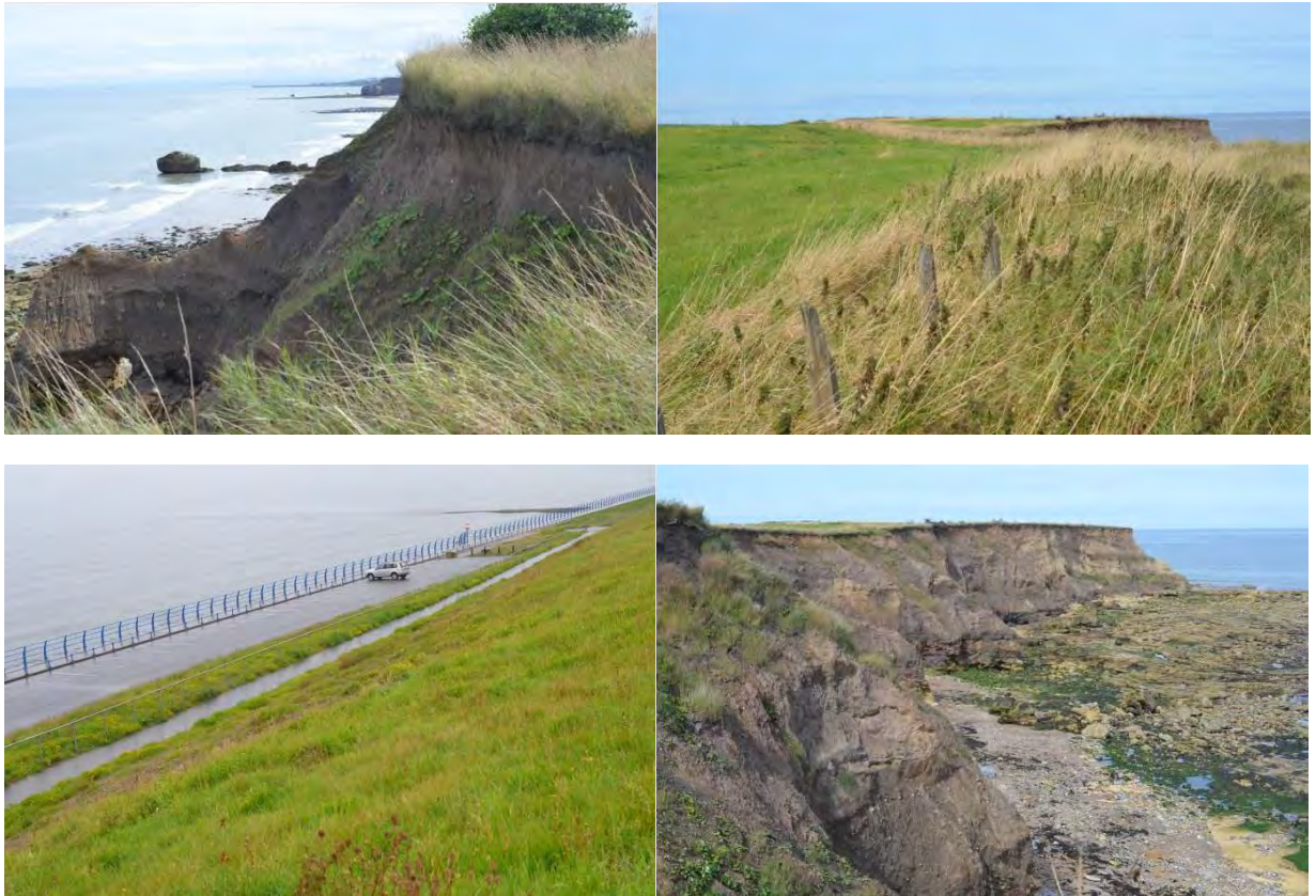
Clockwise from top left: eroding clay cliffs; coastal grasslands; coastal view at Ryhope Nook; car park at Hendon Beach.
