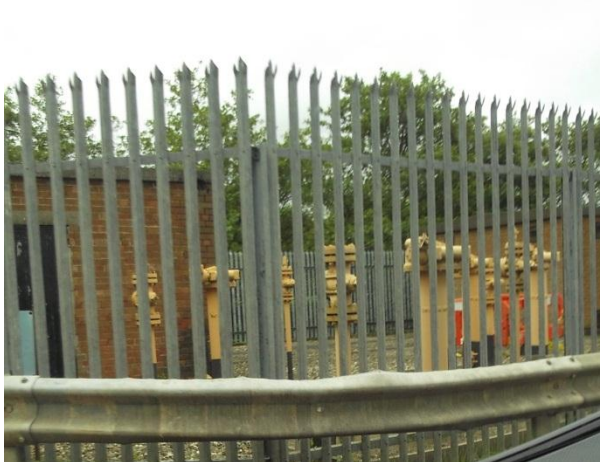
Figure B.26: Gas Valve Compound adjacent to Hylton Grove Farm
