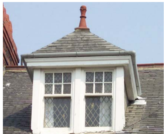
An original dormer feature with timber sliding sash windows, a Welsh slate roof and a terracotta finial to the top, repeated along the terrace at Cedars Gardens
