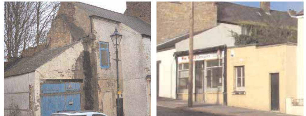
Left: this building has been deteriorating for some time and is in need of some repair work; right: a small cluster of relatively modern flat roofed buildings create a contrast against the historic properties of Nesham Place; these properties could benefit from improvement works
