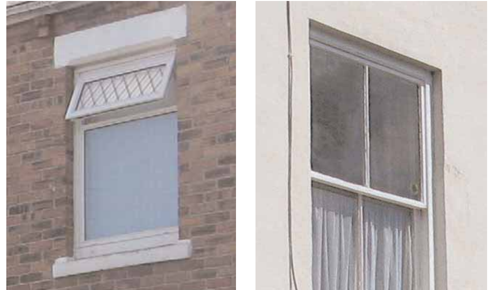
The replacement uPVC window to the left fails to match the slender proportions and historic detailing of the traditional sliding-sash in the property to the right. Such alterations are inappropriate for historic buildings and contrary to the aims of the Article 4(2) Direction.
